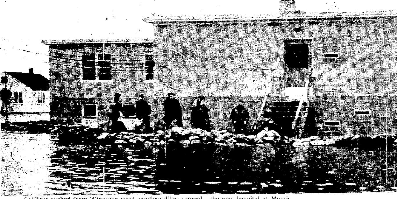
Soldiers rushed from Winnipeg erect sandbag dikes around the new hospital at Morris
